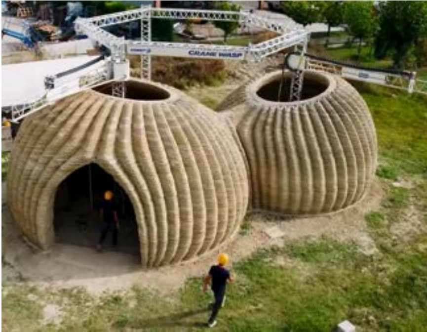
Figure 5: TECLA house: 3D printed residential structure made of clay Milano, A. (2021). Eco-sustainable 3D printed house "Tecla".jpg [photograph]. Wikimedia Commons. https://upload.wikimedia.org/wikipedia/commons/b/bb/Eco-sustainable 3D printed house %22Tecla%22.jpg
