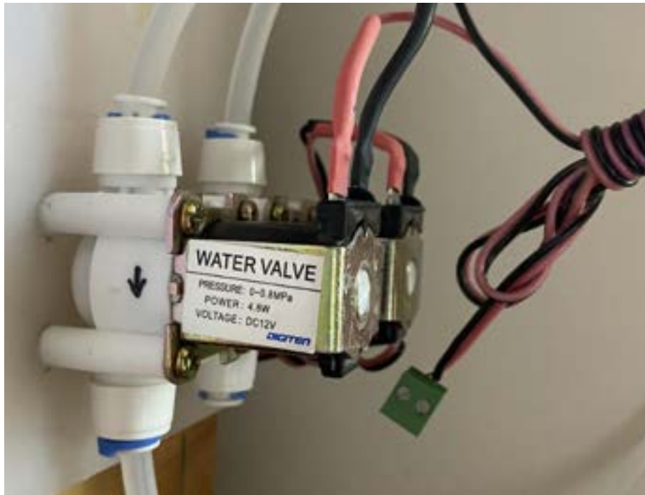
Figure 6: Shown above is the ball-motor valve attached to the PVC watering system.
