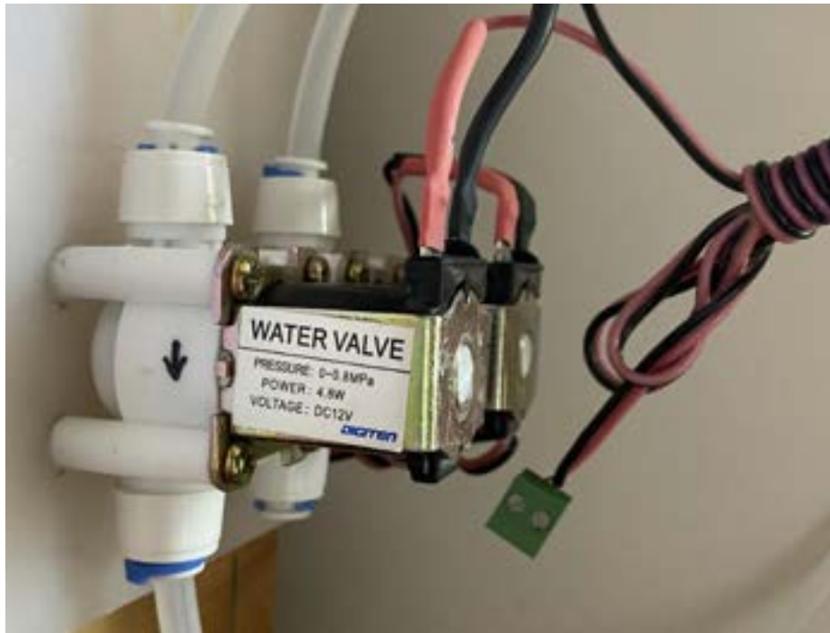
Figure 6: Shown above is the ball-motor valve attached to the PVC watering system.
