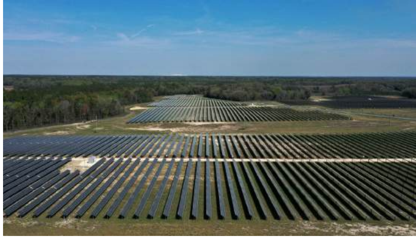
Image from https://flatlandkc.org/news-issues/every-to-lead-group-building-massive-kci-solar-farm/ The solar array systems currently under construction. This is how the solar array systems will look when it is completed.
